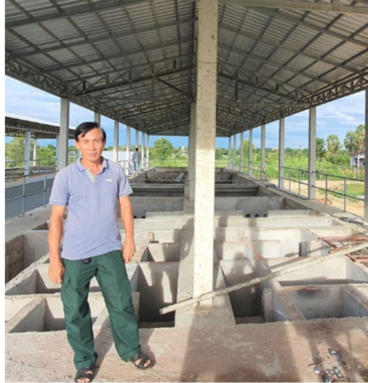
One of the piped water operators we are supporting through the Cambodia Revenue Finance Facility at the construction of his water station.
